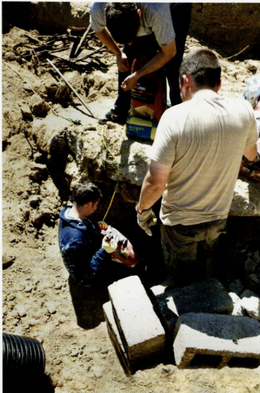
Rob Smith, Adrian and John using the new hole to pass heavy materials into the bunker and avoid a very long barrow run before the pipes are fixed in place.
